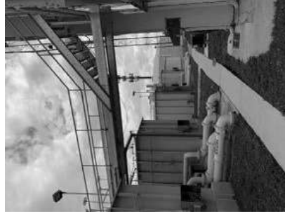
Tamarac Control Building & Water Treatment Plant -CPZ
