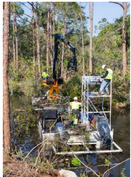
Ceres crew on a barge removing waterway debris in Cape Coral, FL following Hurricane Ian in 2022. Over the course of this large-scale project, Ceres removed a total of 2.7 million cubic yards of debris, both on land and in waterways.
