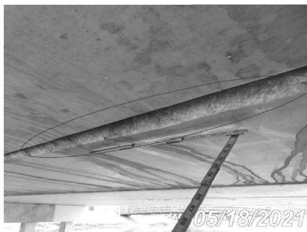
Photo 8099-S01 (Unit 0: PS Conc Slab (Sonovoid)) Spall in the north edge of Slab Unit 1-5, 10ft from End Bent 1
