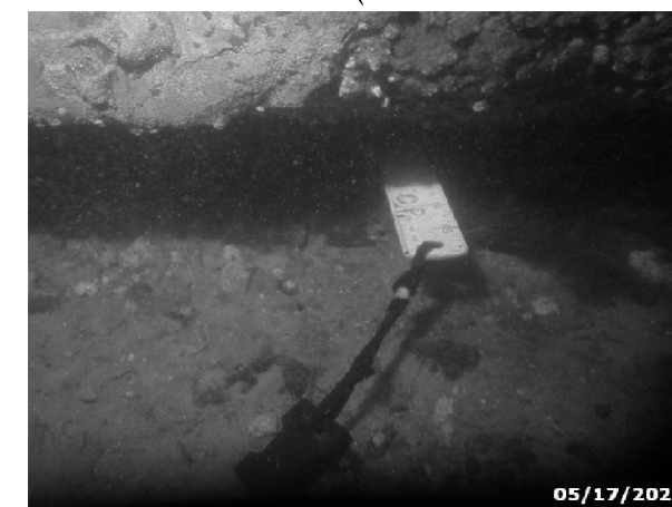
Photo 8290-U01 (Unit 6: Channel) reas of undermining at the east slope protection.
