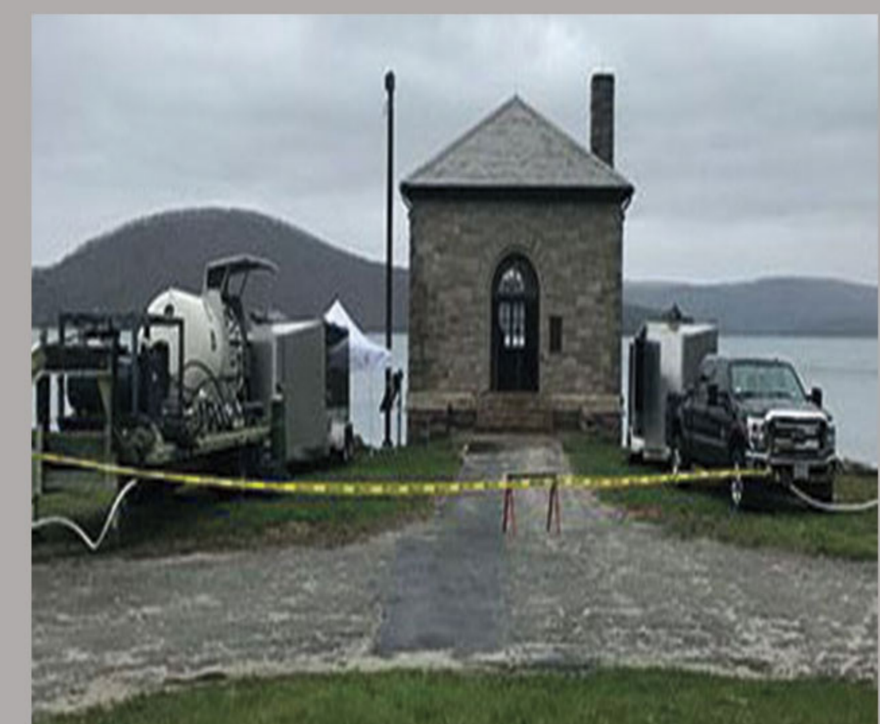
Additional Raw Water Services
