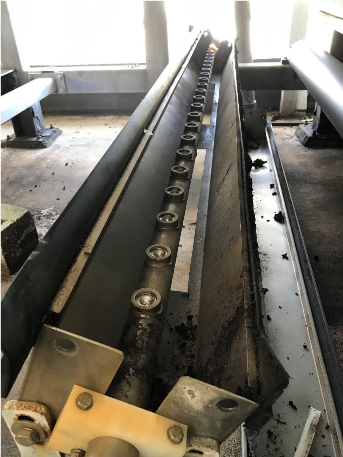
New high pressure spray nozzles installed
