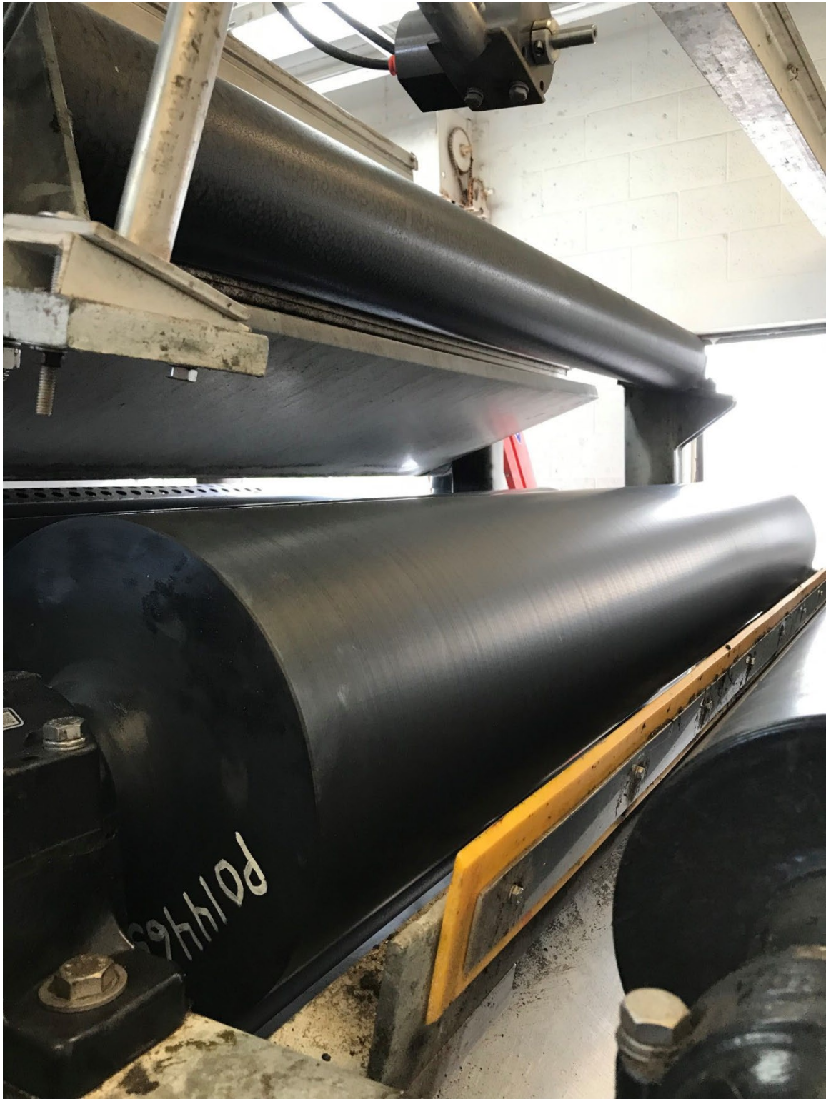
New main drive roller assembly with new bearings installed
